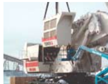
Oil cooler module is mounted on frame
